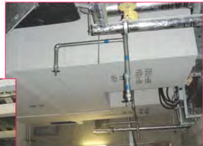
Fire rated duct
