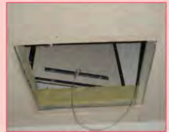
Access panels at fire rated ceiling
